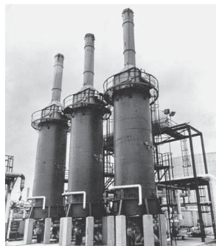
Liquid Asphalt Heaters
