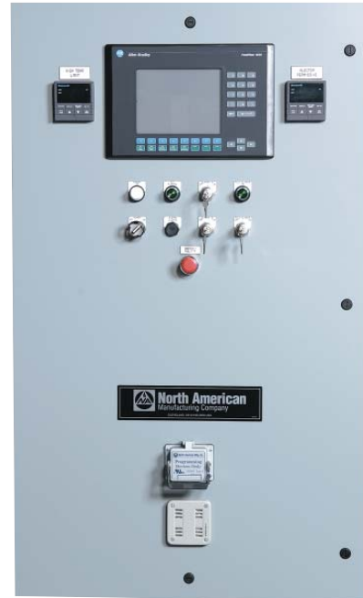
PLC/OIT based combustion safety and process control system.
