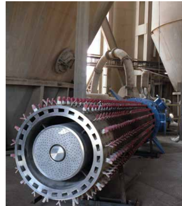
Pillard PrecaFlam™ burner with inlet to feed coarse alternative fuels.
